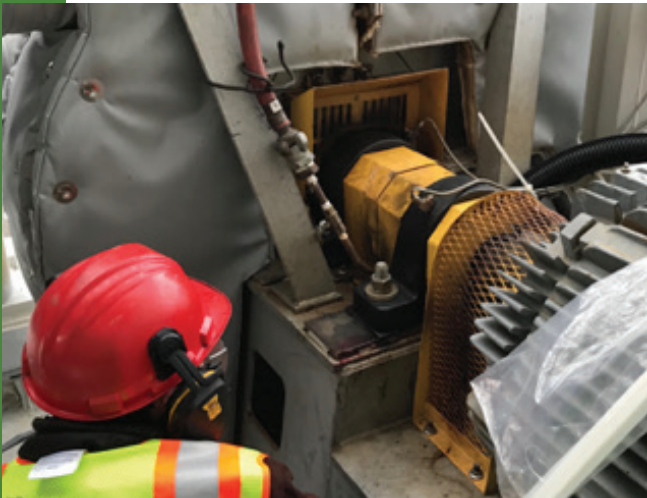
An inspection is conducted by a technician to determine the cause of overheated bearings.
