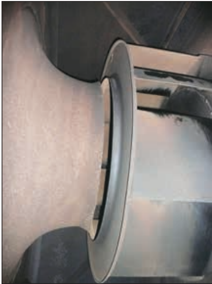
Figure 4: An incorrect setting of the inlet cone to the impeller.
