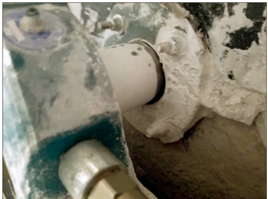
Figure 3: A worn fan shaft seal.
