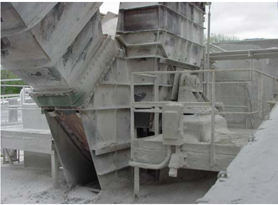
Example of buildup around fan unit in production facility.
