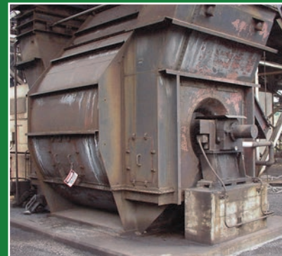
New York Blower Company replacement project which included replacing wheels, inlet pieces and portions of the housing.
